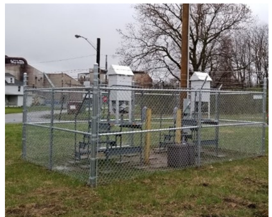
Republic Steel Community air monitoring site for lead and metals at Marietta Ave. NE & Georgetown Rd.
